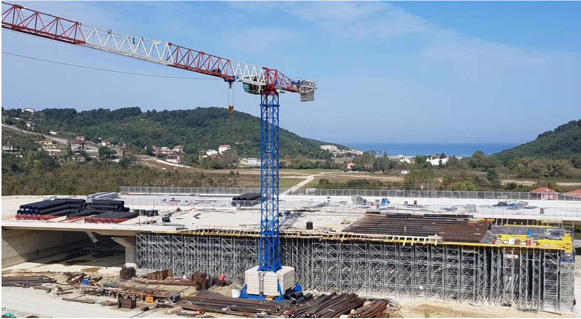
In July 2022, Kalyon and Makyol Groups won a 5.7 billion lira contract to build two highways outside of Istanbul. Construction of one of these, the Şile-Ağva highway (shown above), began August 15, 2022. Photo credit: Intek Formwork and Scaffolding
